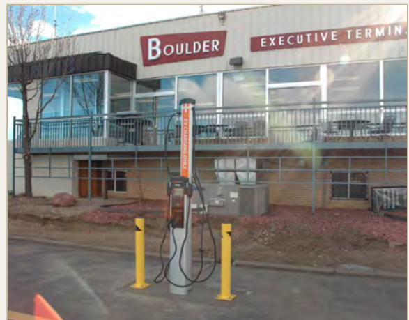
Electric aircraft charging station now in service at KBDU.
